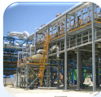
Dry Cooling Systems
