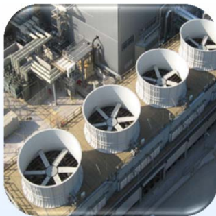
Wet Cooling Systems
