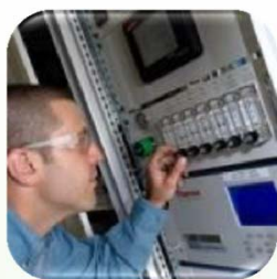
Air Pollution Control Systems
