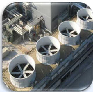
Wet Cooling Systems
