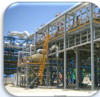
Dry Cooling Systems
